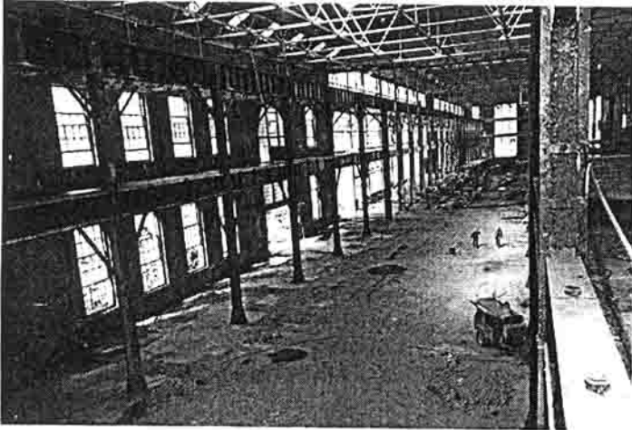
Fig. 9 Building 42 craneway 700 ft. long with side galleries (looking north from 42A to 42S & 42N).
